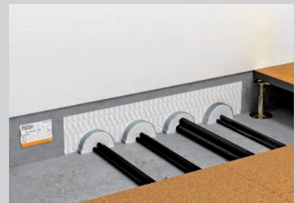
Fully installed half shell in PYROPLATE® Fibre soft insulation.
