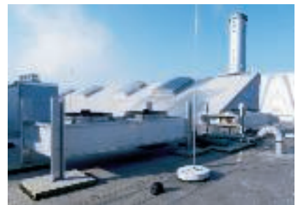
Insulated lightning protection on roof fitments
