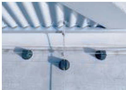
A metal facade connected to the lightning protection system
